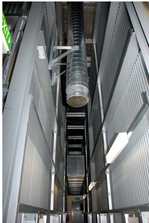
Figure 4: Fumigant extraction tubes located in the return air and exit corridors
