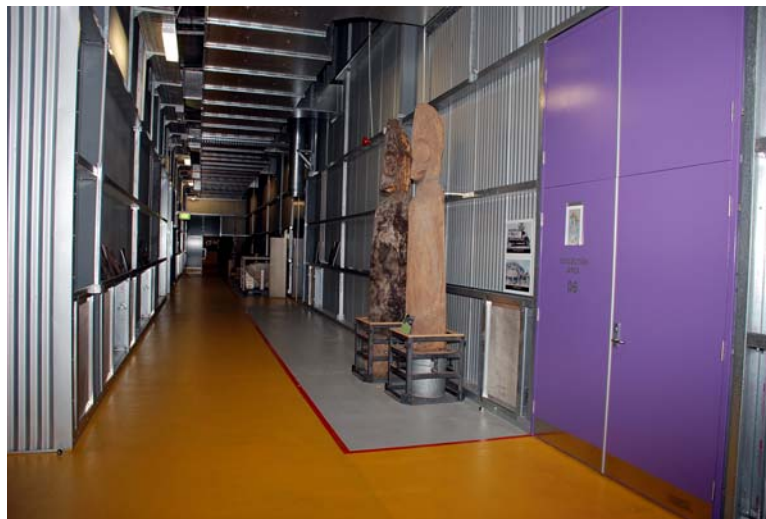
Figure 6: Corridor in the main collections building showing viewable storage and air-conditioning supply ducts.
