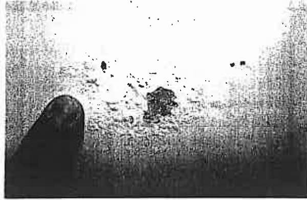
Figure 6. Filiform corrosion on the mast of Australia II , prior to stripping and repainting.
